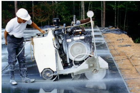
Water used to cool the blade of a concrete cutter like this can carry pollutants to storm drains.
