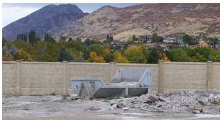
A concrete washout bin. The company will haul this for proper disposal at a later date.
