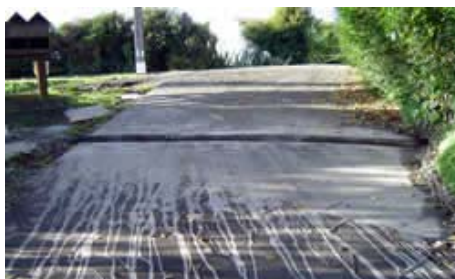
Not cleaning up from concrete cutting can lead to scenes like this.
