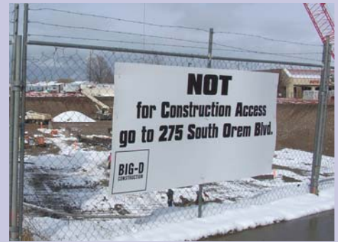
Chain link fence is often used to control access to construction sites
