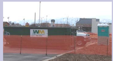
Caution should be taken when placing trash bins and portable toilets
