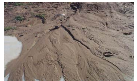
A silt fence could have kept this dirt from leaving this site
